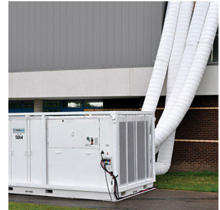
Temporary HVAC system Source: www.esmagazine.com
