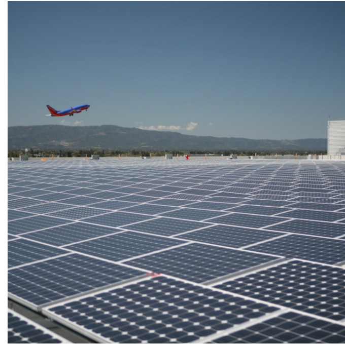
Rooftop solar panels at Cochin International Airport Source: www.newsaurchai.com
