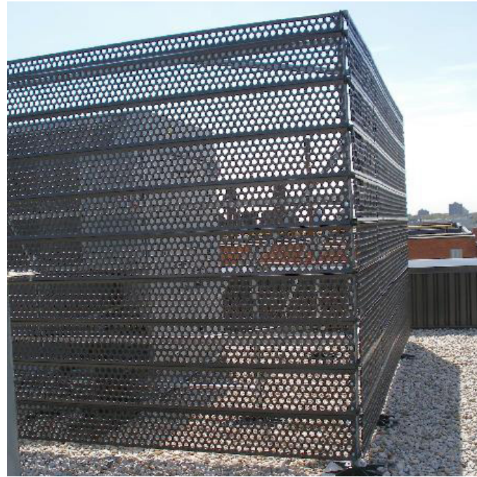
Rooftop HVAC equipment screens with Zero Roof Penetration. Source: www.planthub.com/
