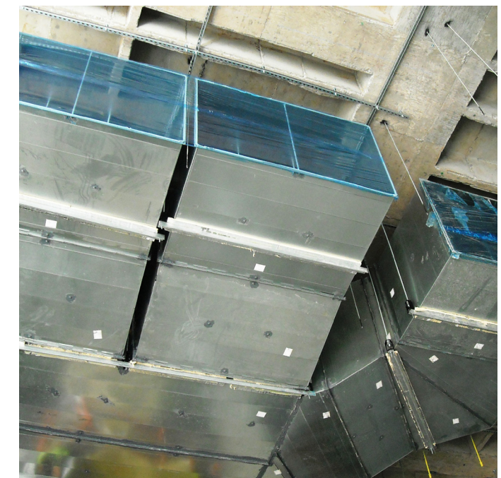
Covered duct openings Source: www.ky.gov
